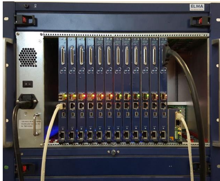
Figure 2. Customized MicroTCA chassis hosting 12 UDSPT boards
