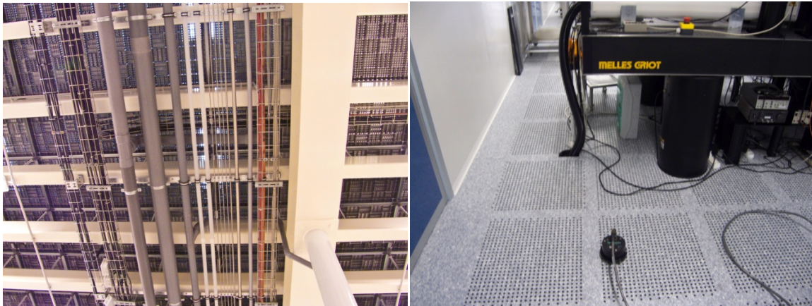
Figure 8: The Episensor installation at FLO1 (floor of the first floor clean room).
