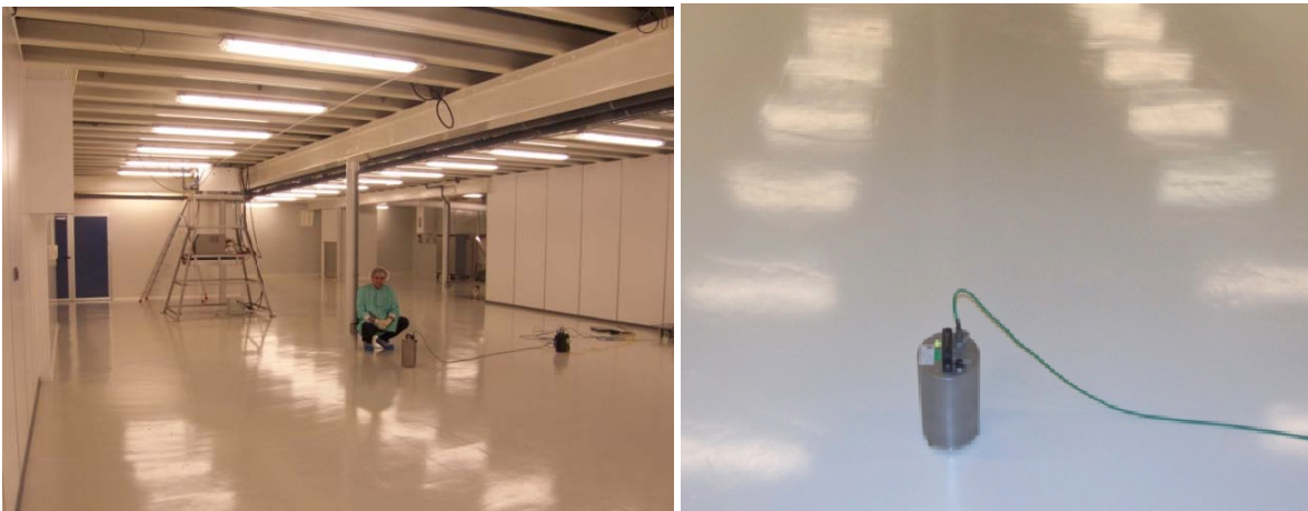
Figure 4: The Guralp installation at LMA building ground zero. The Guralp “North arrow” is perpendicular to and points towards the end wall located on the left when entering the room.
