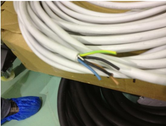
(Figure 1) These wires contained in the high voltage power cables are used to power most of the Virgo infrastructure. Three of the cables are used to transmit the three-phase current while the fourth acts as a “neutral” wire sending a reverse current whose amplitude in time is the sum of the three phases while a fifth wire acts as ground.
