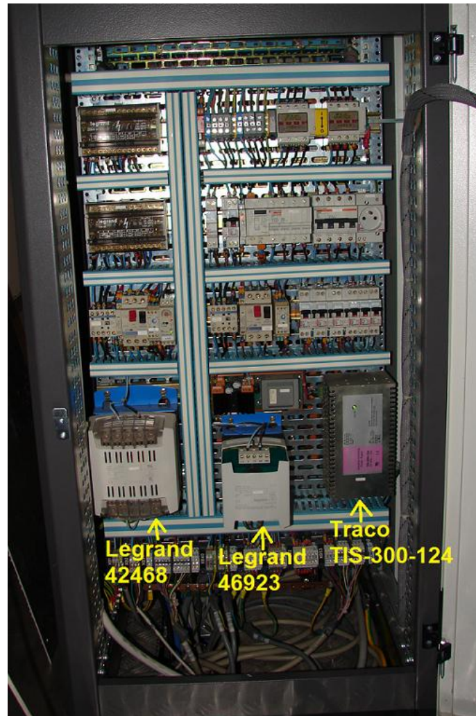
Figure 1a. Tower Vacuum Rack.
