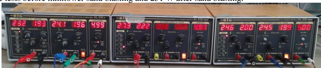
Figure 9 Reading of the power supply for the April 11 test .The 24V or so are used to power the resistors. The 5V are used by the temperatures probes.
